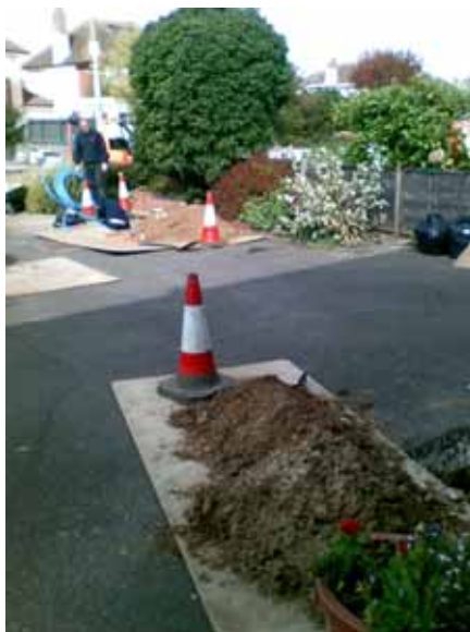
The driveway in Christchurch beneath which the new water pipe was installed using the HammerHead impact mole.
