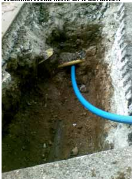
The new 25 mm diameter MDPE pipe being installed behind the HammerHead mole as it advances.
