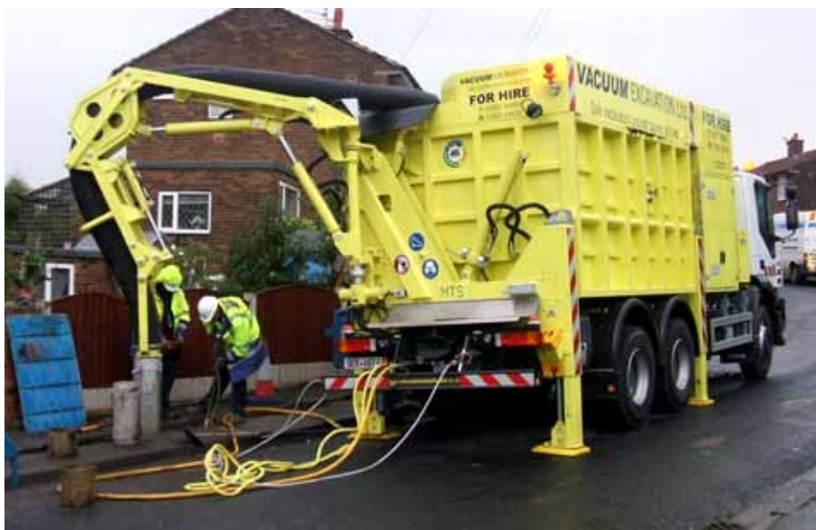
A Dino III vacuum excavation unit in operation with Vacuum Excavation Ltd.
