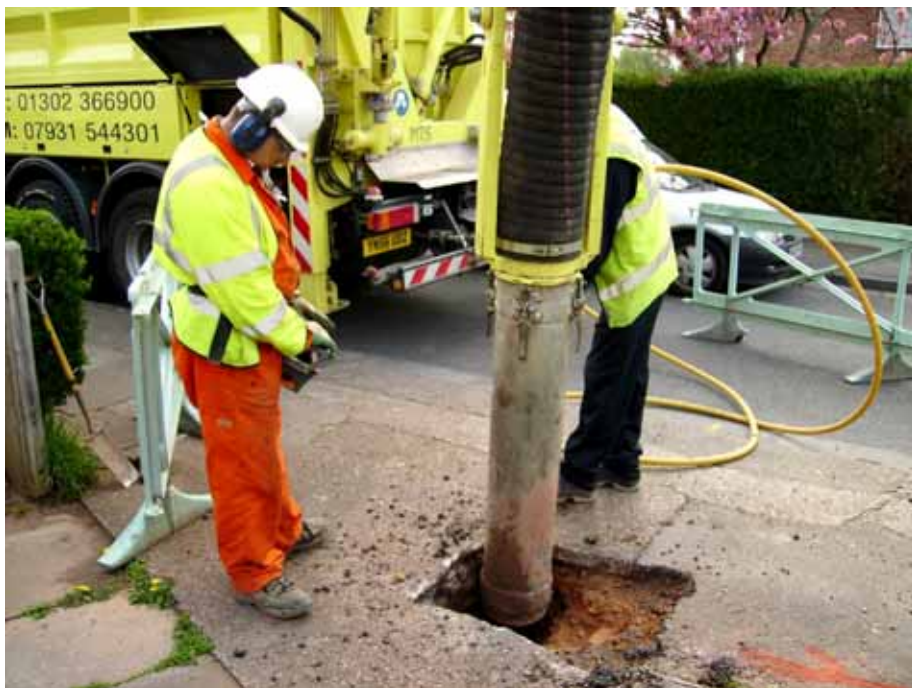
Utilities can be excavated with precision and without damage when using vacuum excavation.
